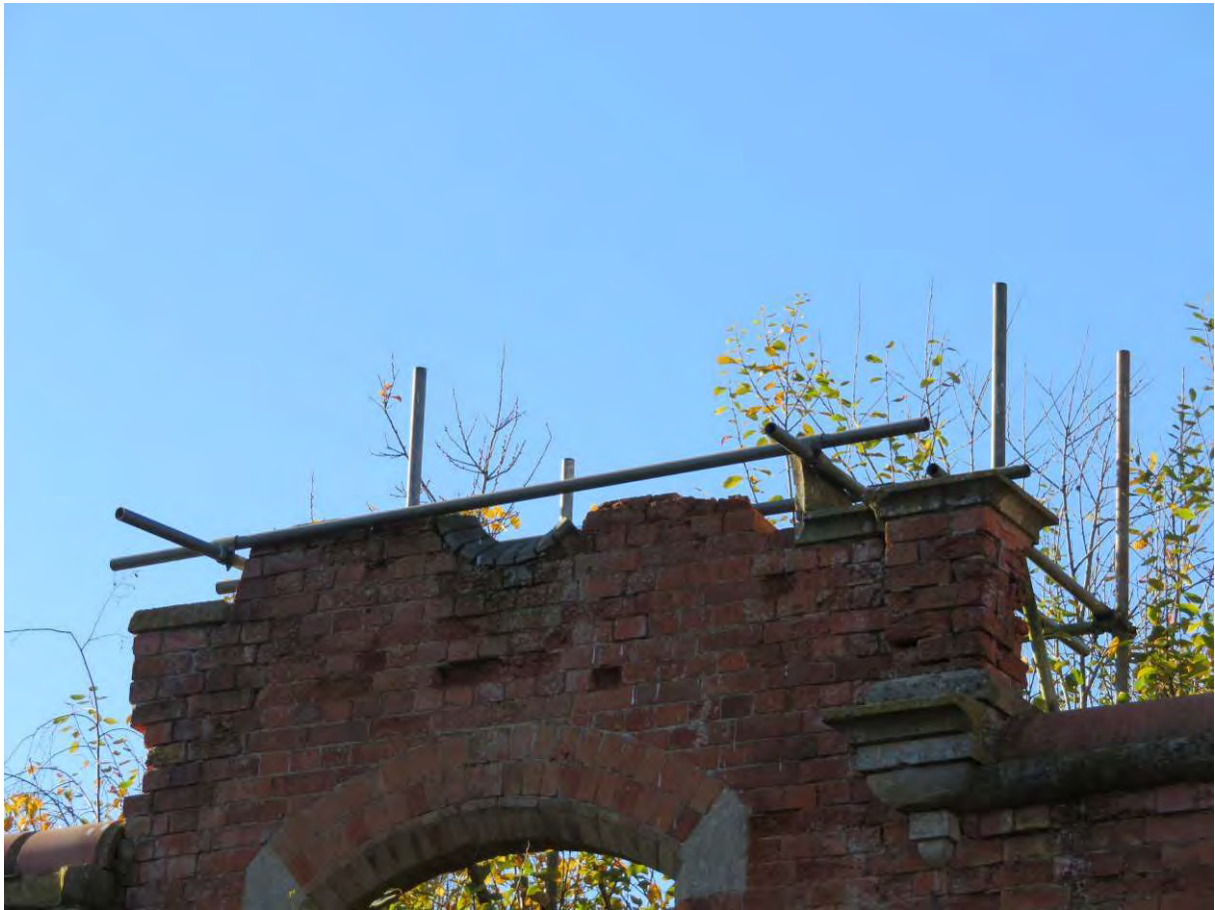
Photograph 27: Lost head to pediment to east side of Room 3
