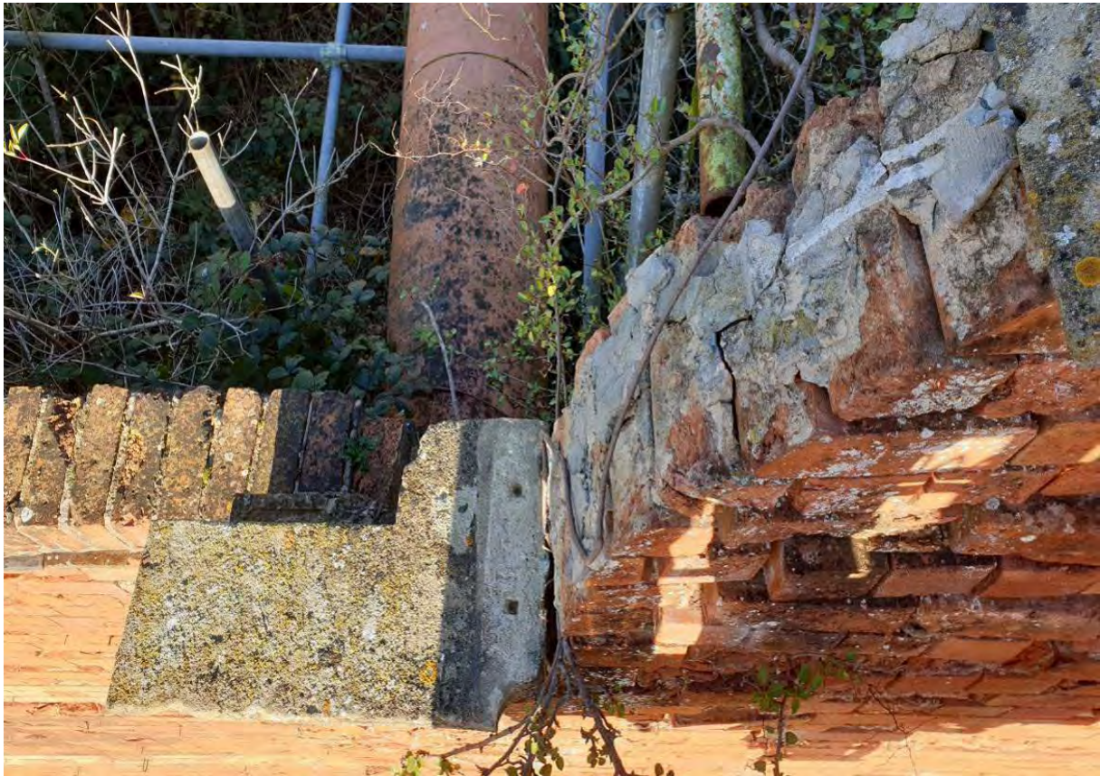
Photograph 11: Missing coping stone to the east end of the south elevation (south range)
