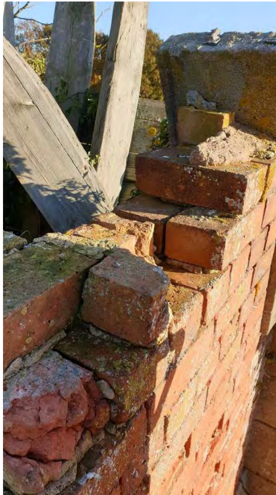
Photograph 7: Loose bricks at timber roof base level - south range tower
