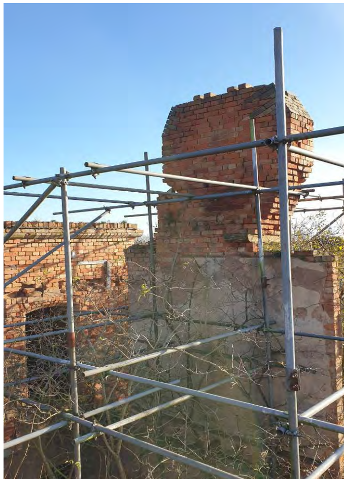
Photograph 18: Stepped chimney stack to be inspected from close-level, and to be provided with temporary support, as appropriate (east range)
