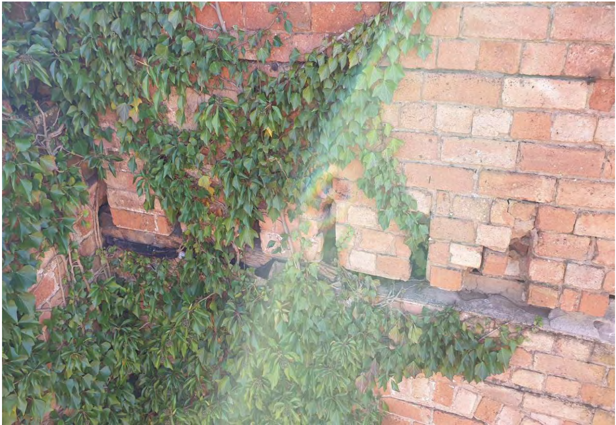
Photograph 15: Embedded timber plates rotten away (north range)
