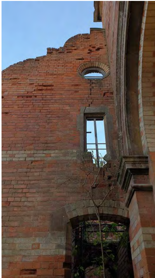
Photograph 41: Cracks over openings towards Room 20c
