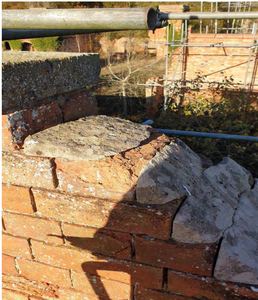
Photograph 10: Deteriorated coping stone noted to the east end of the south elevation
