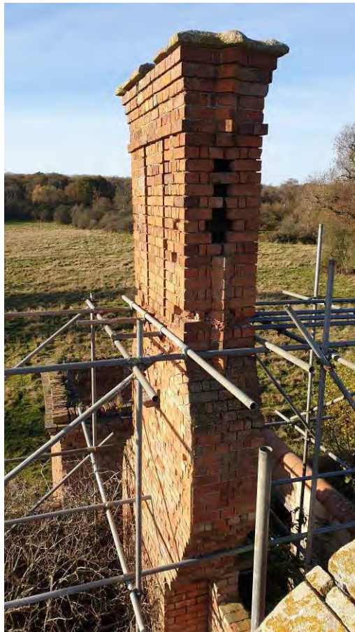
Photograph 54: Chimney to Room 4 with missing bricks
