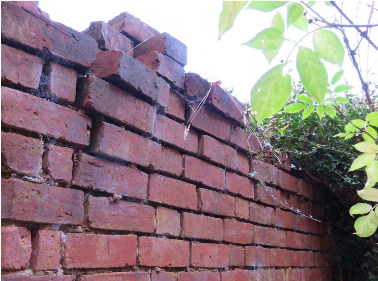
Photograph 58: Kennels brickwork on poor condition
