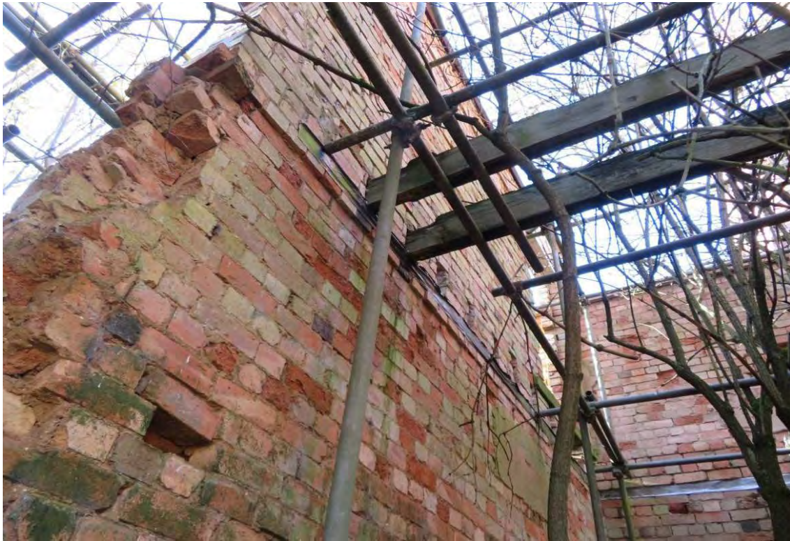
Photograph 21: Bonding timber acting also as a wall plate providing support to joists. Vulnerable area for the 9 inch cross wall in question.
