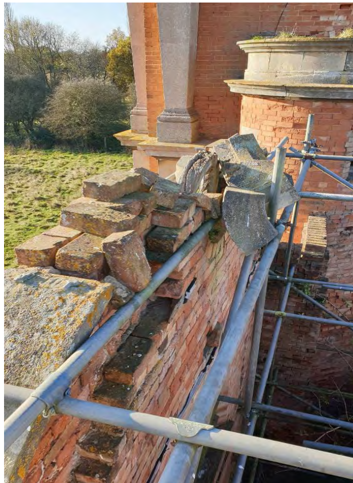
Photograph 12: Collapsed stone dressings to the south elevation of the south range
