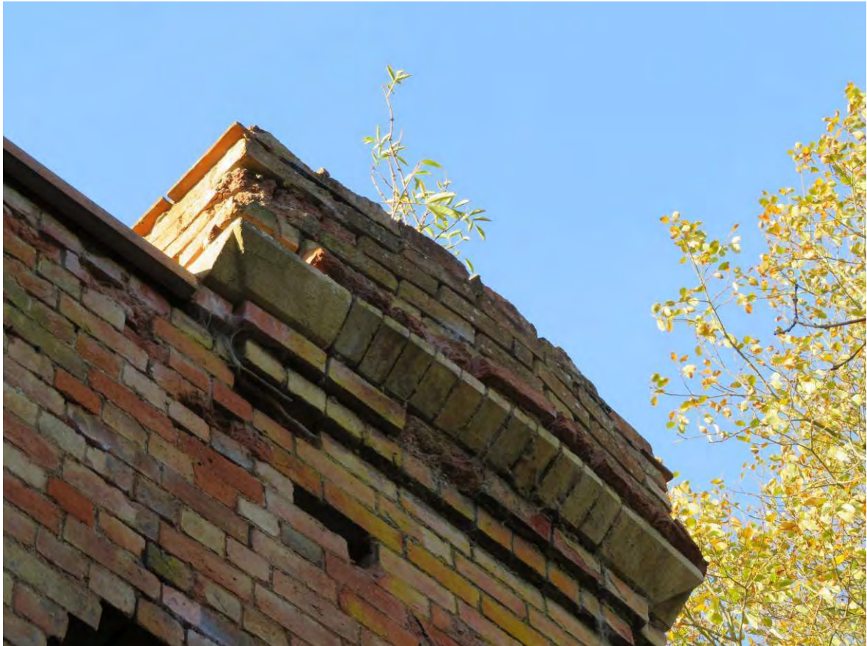
Photograph 34: Bulged chimney to west elevation to Room 10a
