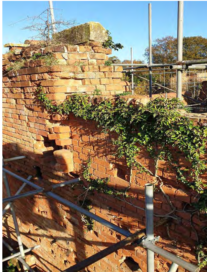
Photograph 13: Climbing plants overgrowth to the south range
