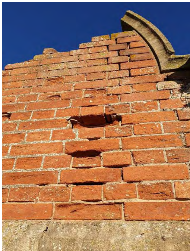
Photograph 8: Eroded bricks at upper stage of tower - south range south elevation (south range)
