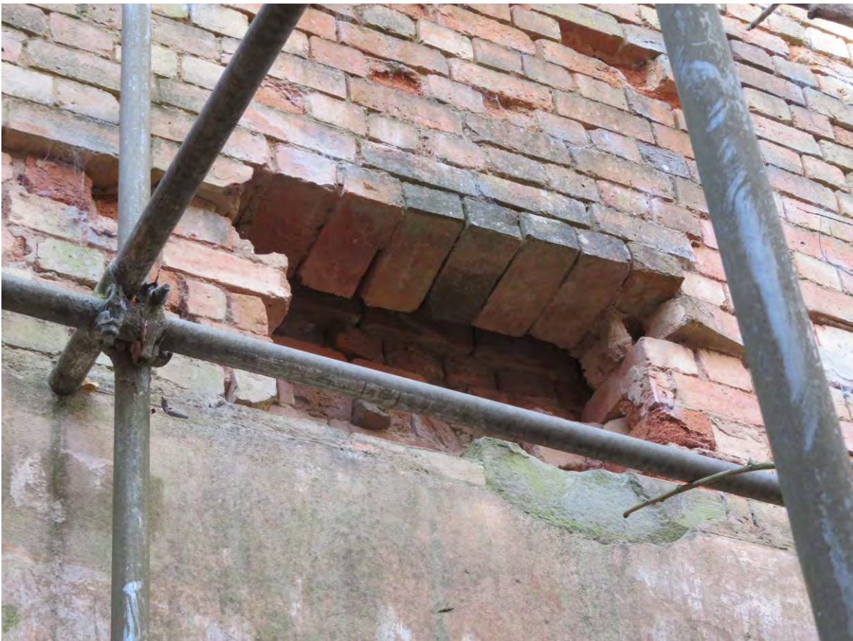
Photograph 26: Room 3 west wall hole
