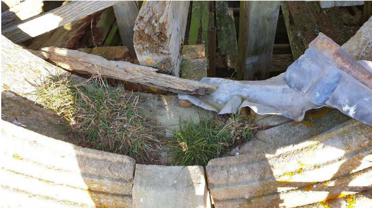
Photograph 48: Loose timbers, leadwork etc.
