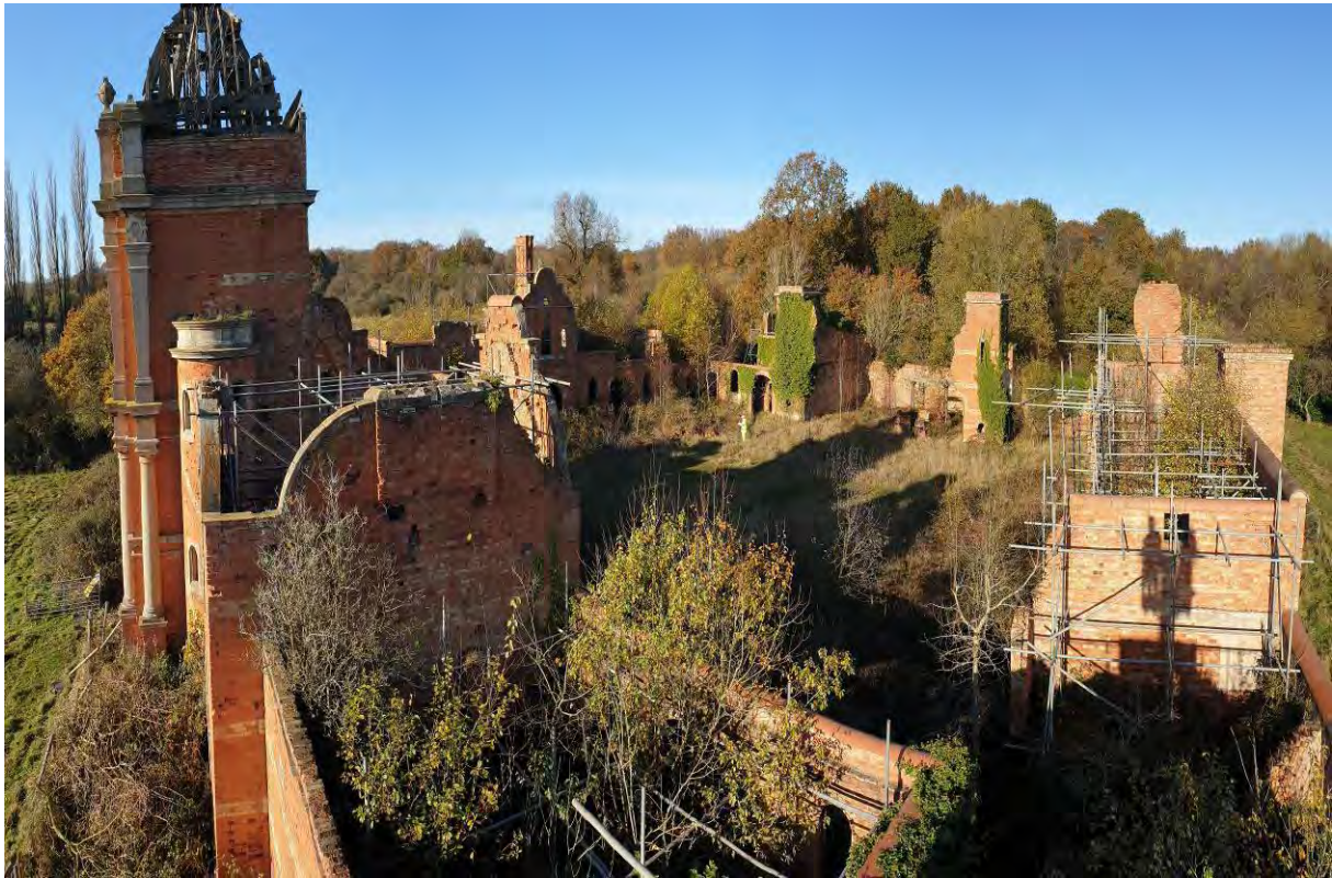
Photograph 9: Vegetation overgrowth throughout the stables and kennels, as seen from cherry picker
