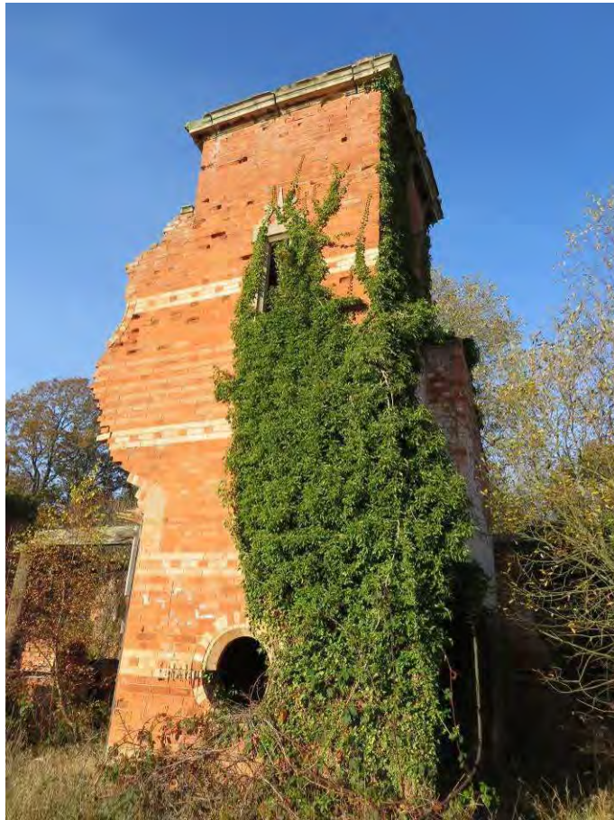
Photograph 33: Eroded mortar joints to tower head to Room 10
