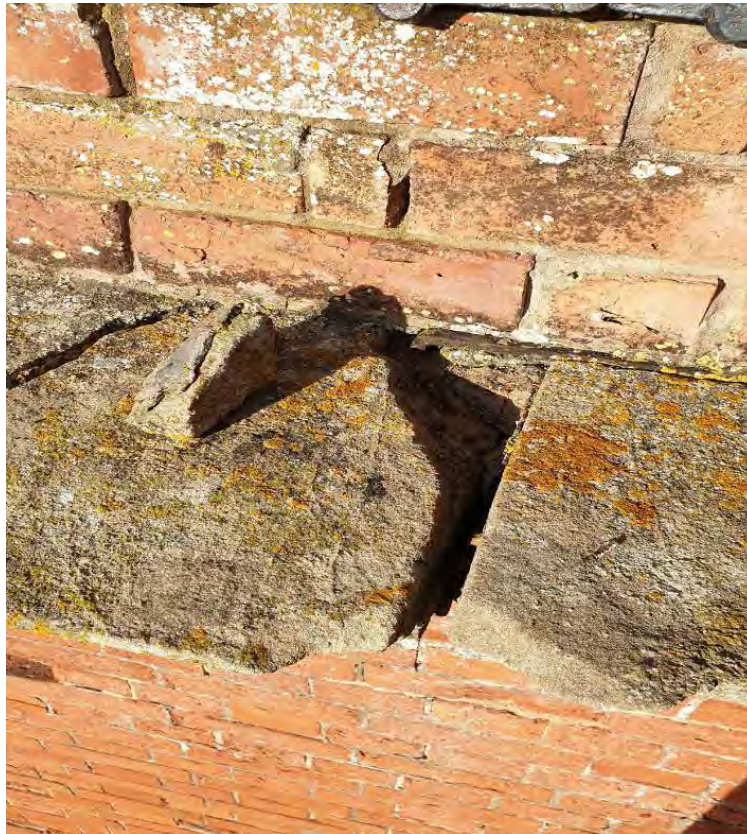
Photograph 17: Damaged and loose coping stone at high level (north range - area '10')
