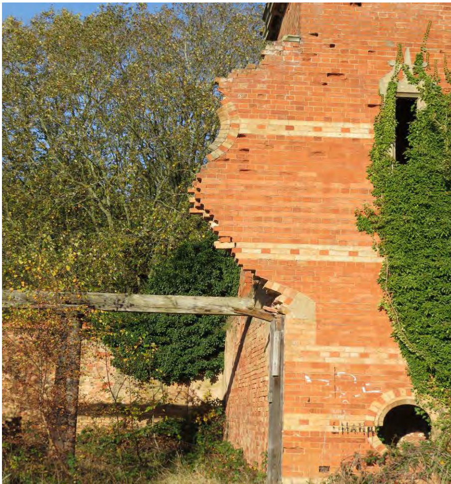
Photograph 22: Loose bricks and lack of adequate support to the south wall of area '9' (north range)
