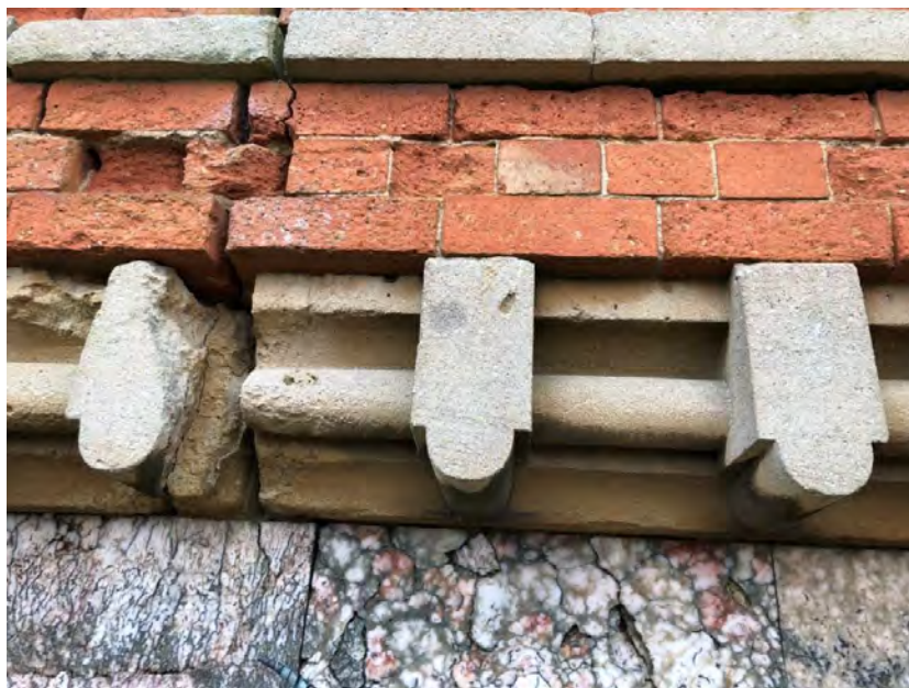
Plate 17: Cracking in the masonry above the panel leading to openings for water penetration.
