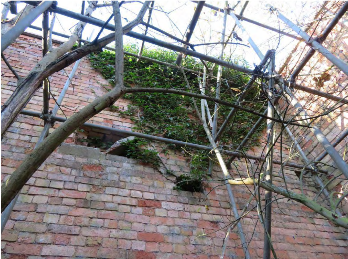
Photograph 30: Hole in rear wall of Room 5
